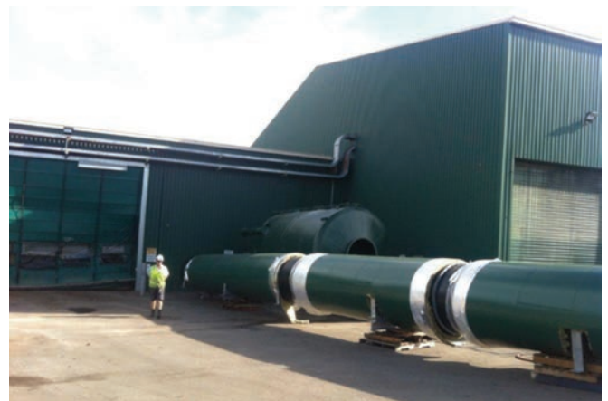
This photo shows Humidifier 4 and ductwork ready to be lifted into position on Bio Filter 1.
