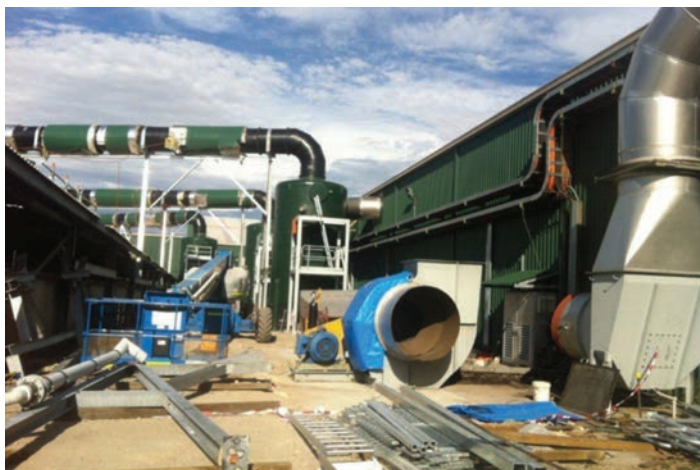
This photo shows the fan area prepared for the installation of Humidifier 4
